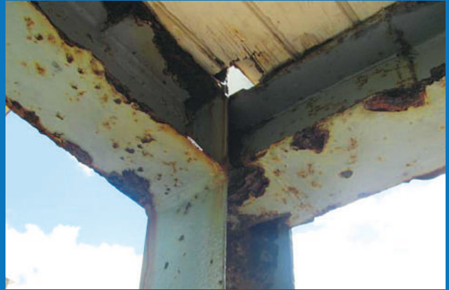
■ CORRODED STRUCTURAL STEEL MEMBERS
