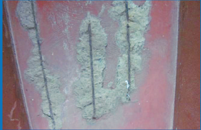
■ EXPOSED CORRODED STEEL REINFORCEMENT IN FLOOR SLAB
