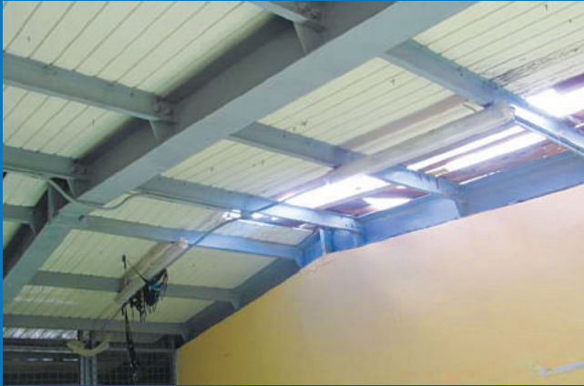
■ SECTION OF SCHOOL NOT IN USE DUE TO HURRICANE DAMAGE
