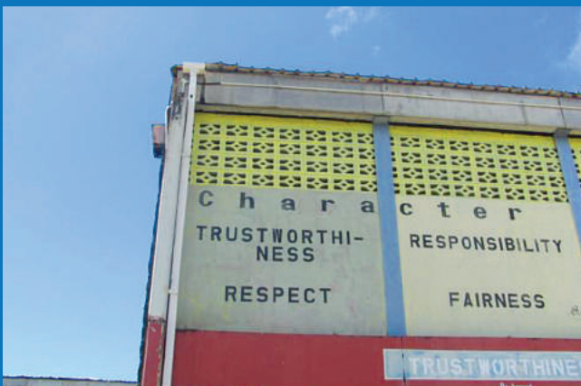
■ ROOF DRAINS DESTROYED BY HURRICANE, MARIA IN 2017
