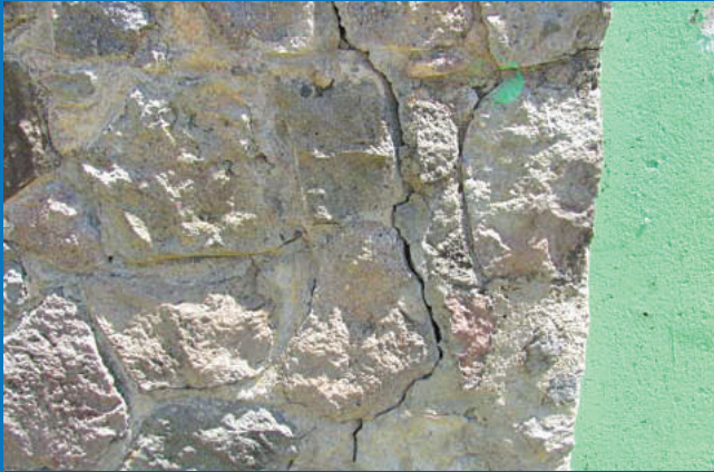
■ CRACKS IN STONE MASONRY WALL
