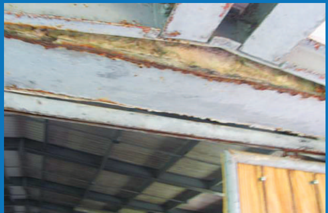
■ CORRODED STRUCTURAL STEEL MEMBERS
