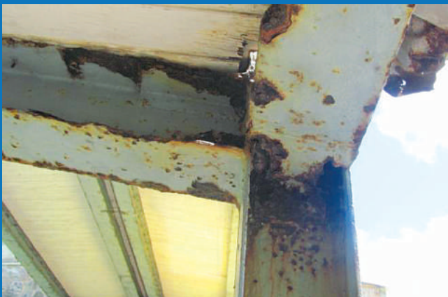
■ CORRODED STRUCTURAL STEEL MEMBERS
