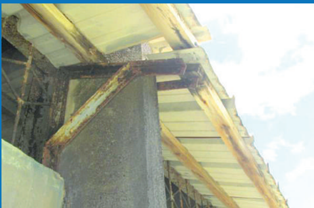
■ CORRODED STRUCTURAL STEEL MEMBERS
