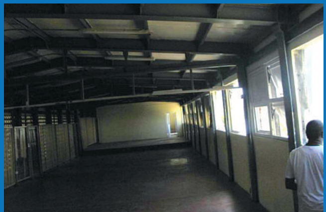
■ SECTION OF SCHOOL NOT IN USE DUE TO HURRICANE DAMAGE TO ROOF AND WINDOWS
