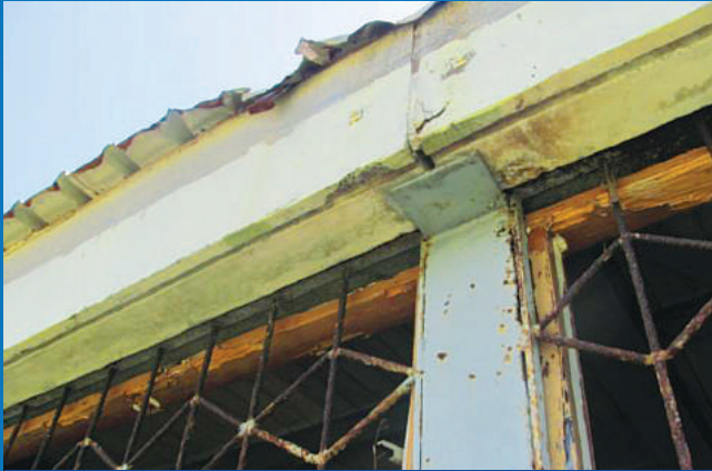
■ CORRODED STRUCTURAL STEEL MEMBERS
