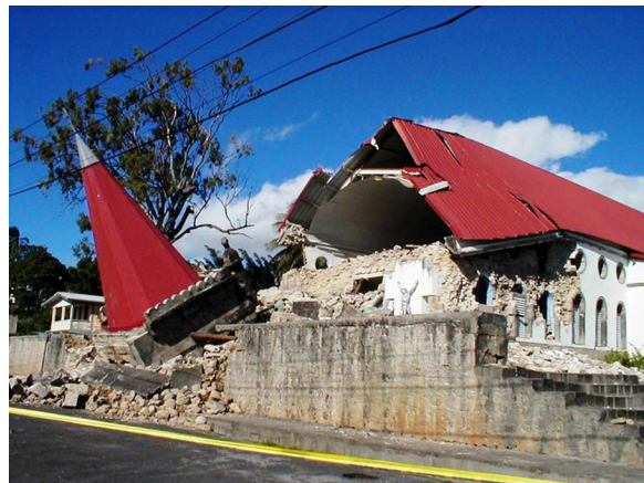
Structural damage caused by the Nov 21, 2004 earthquake with an epicenter just north of Dominica
