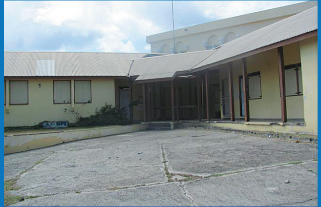
■ BLOCK IN STATE OF DISREPAIR
