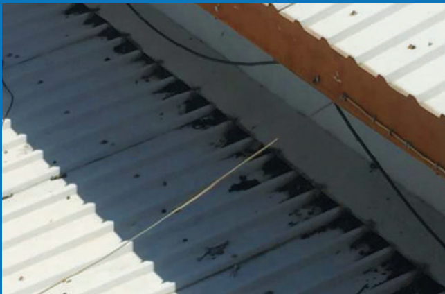
■ EXPOSED ELECTRICAL WIRES
