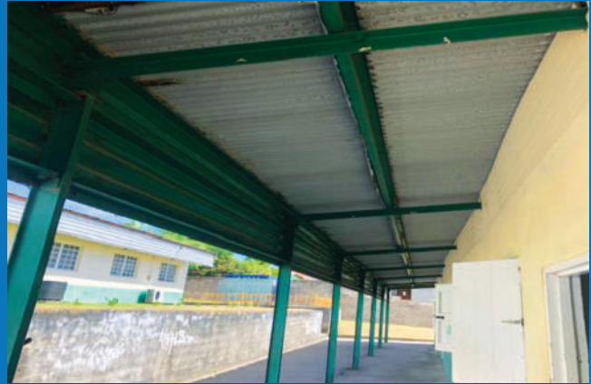
■ STEEL FRAME BUILDING WITH CORRODED ROOF SHEETS
