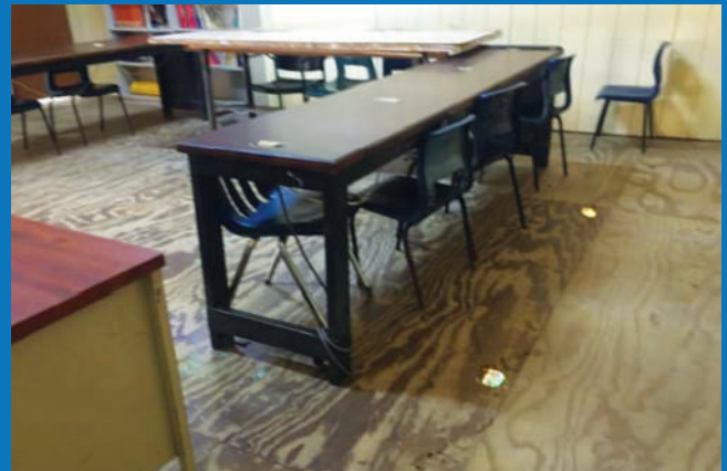
■ TIMBER BUILDING - TERMITE DAMAGE
