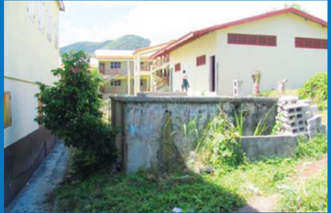
■ CISTERN - IN NEED OF REPAIRS
