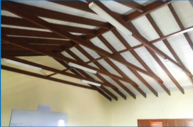
■ TYPICAL CLASSROOM LIGHTING
