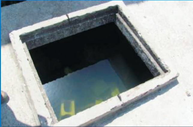
■ CISTERN - IN NEED OF REPAIRS
