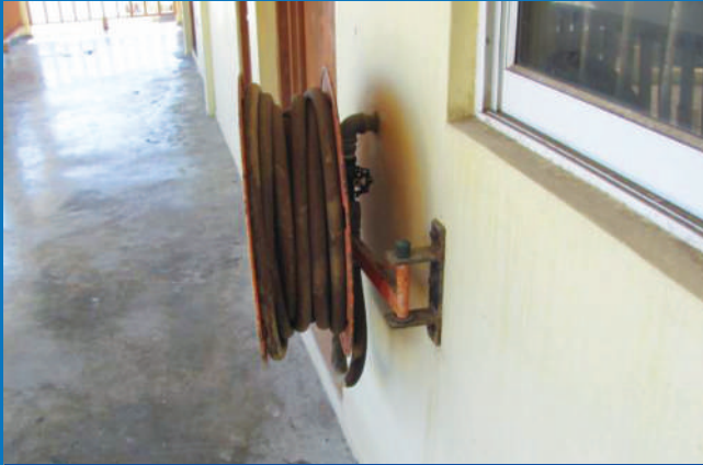
■ FIRE HOSE REEL
