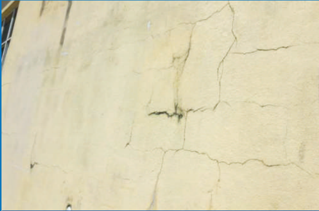
■ SIGNS OF MOISTURE PENETRATION - CRACKS
