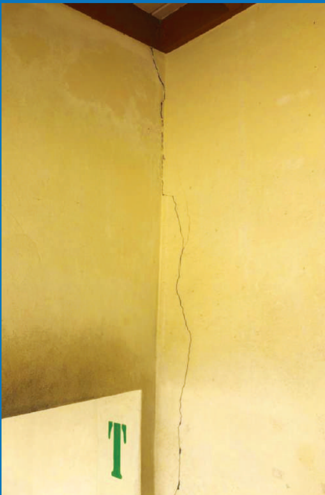
■ VERTICAL HAIRLINE CRACKS TO WALL
