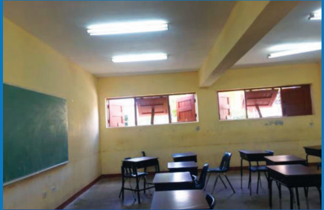
■ TYPICAL CLASSROOM LIGHTING
