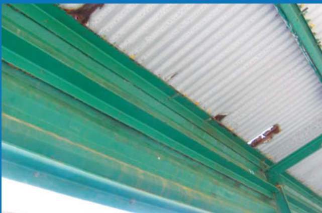
■ CORRODED ROOF SHEETING
