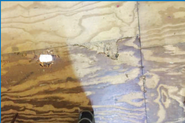
■ TIMBER BUILDING - TERMITE DAMAGE
