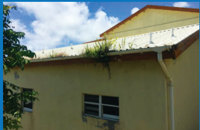
■ ROOF DAMAGE - NEEDS ATTENTION
