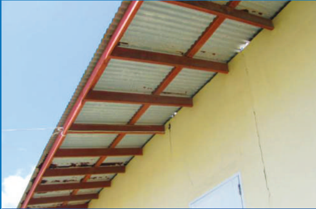
■ LIGHT WEIGHT ROOF IN A STATE OF DESPAIR
