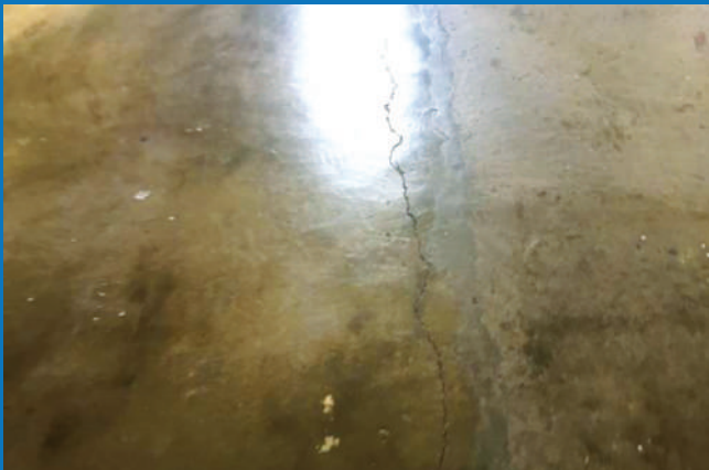
■ CRACKS TO FLOOR SLAB
