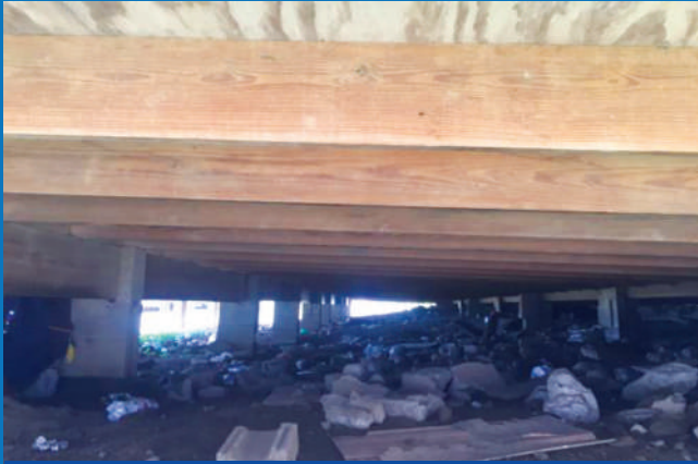
■ TIMBER BUILDING - GARBAGE DISPOSAL AND OTHER SAFETY ISSUES
