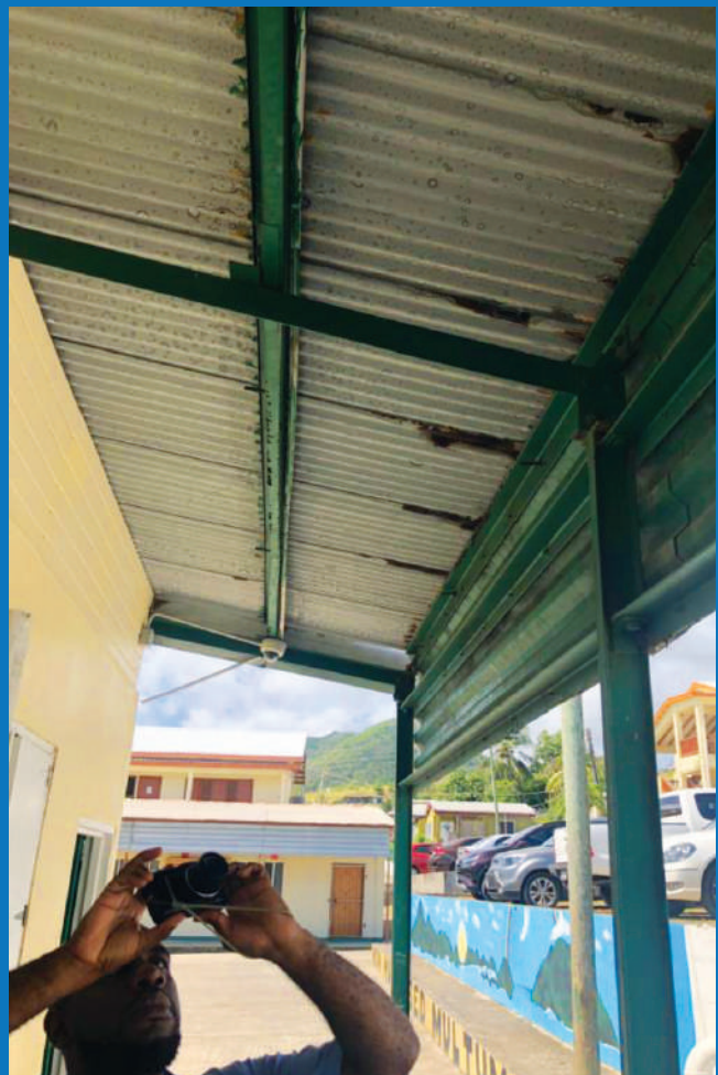
■ STEEL FRAME BUILDING WITH CORRODED ROOF SHEETS
