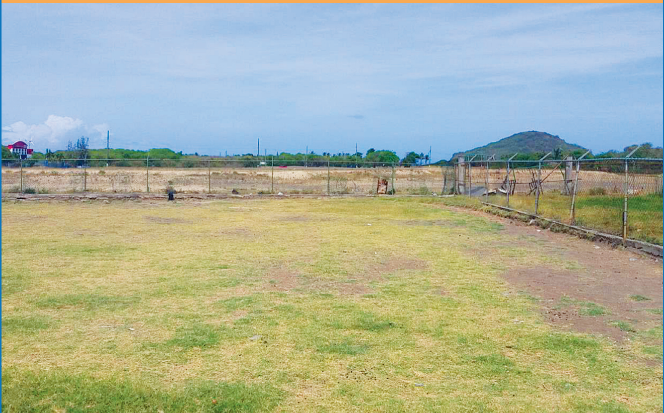
FIGURE 7.2: PERIMETER FENCE IN NEED OF REPAIR AT VIEUX FORT PRIMARY (MAY 2019)
