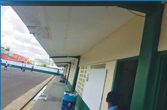
■ WATER DAMAGED CEILING
