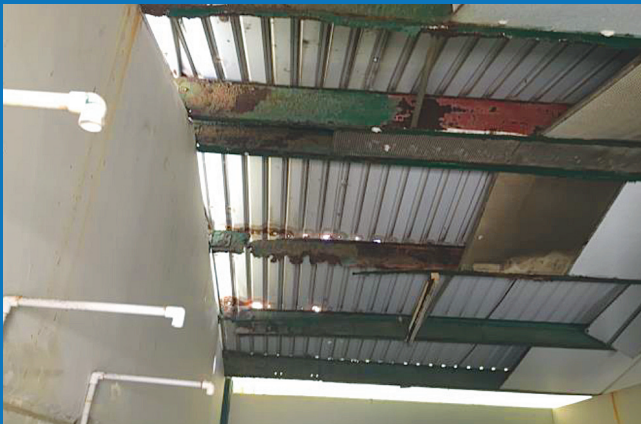
■ CORRODED ROOF STRUCTURE OF TOILETS
