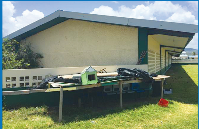
■ TYPICAL END VIEW WITH EXCESSIVE EAVES
