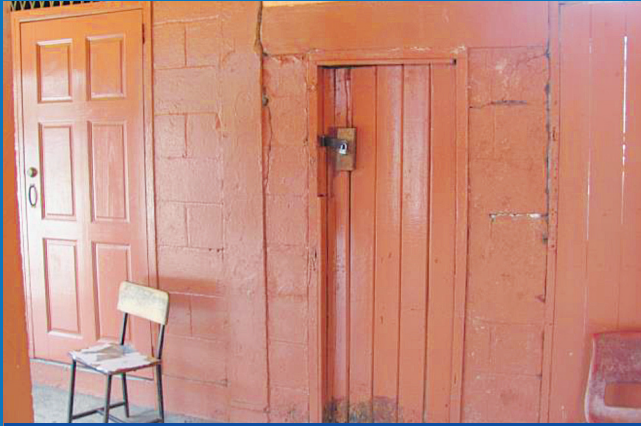
■ STOREROOM IN NEED OF REPAIRS
