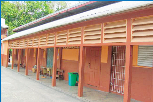
■ BUILDING ORIGINALLY 2-STOREYS TOP FLOOR DEMOLISHED- EXCESSIVE SETTLEMENT WAS OBSERVED
