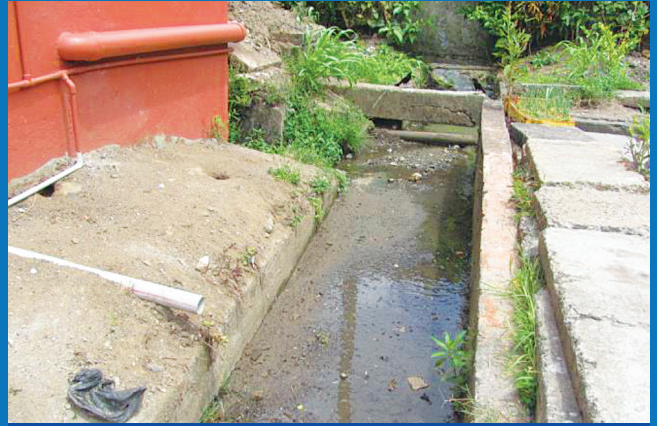
■ STOREROOM IN NEED OF REPAIRS
