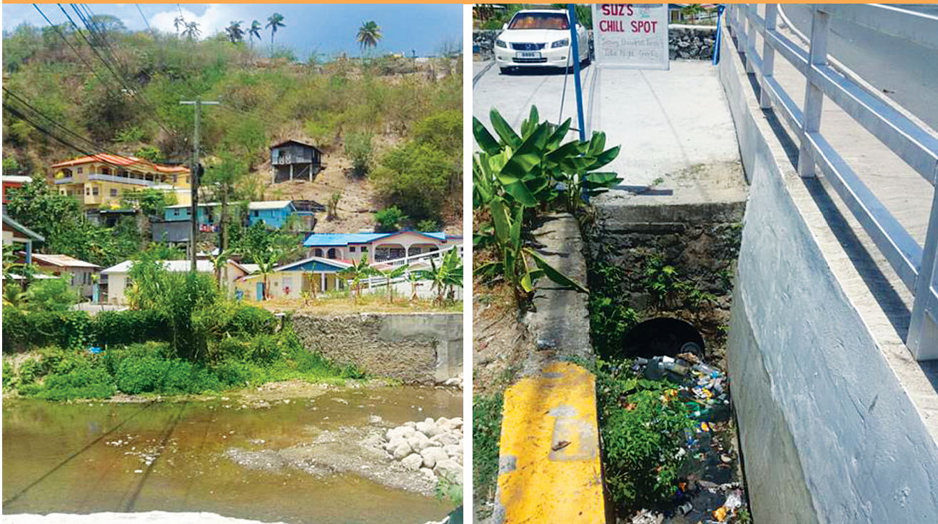
FIGURE 4.2: LEFT: CANARIES RIVER SOUTH OF SCHOOL; RIGHT: SOLID WASTE IN DRAINS THAT MAY EXACERBATE FLOODING
