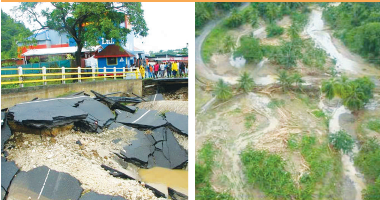
FIGURE 3.1: IMPACTS OF HURRICANE TOMAS (2010). SOURCE: SLU DRR
