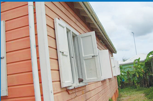
■ TIMBER BUILDING REMAINS VERY VULNERABLE TO HURRICANES
