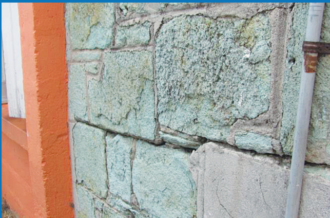
■ DETERIORATING MASONRY JOINTS
