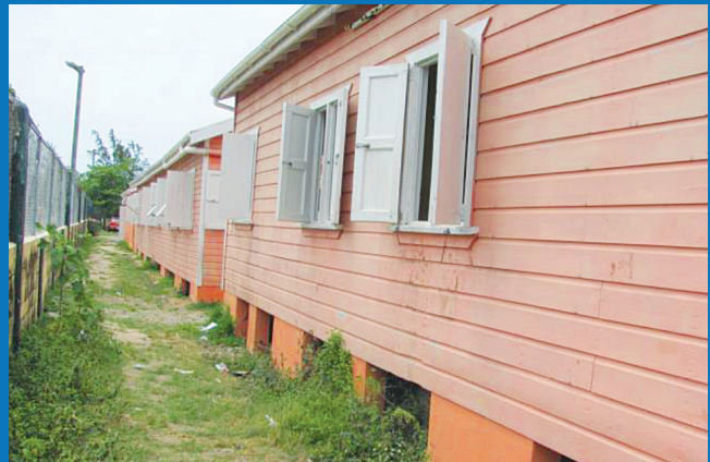
■ TIMBER BUILDING REMAINS VERY VULNERABLE TO HURRICANES
