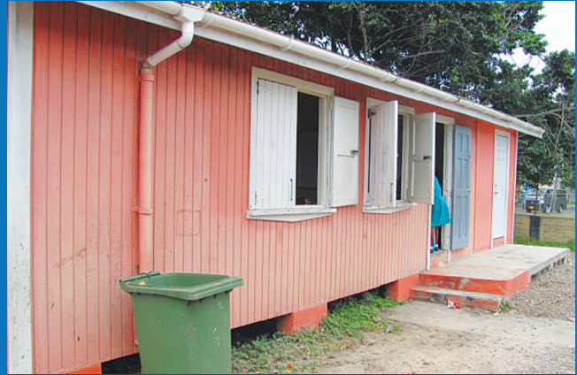
■ TIMBER BUILDING REMAINS VERY VULNERABLE TO HURRICANES
