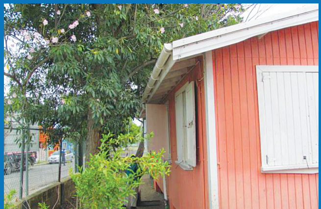
■ TREE IN CLOSE PROXIMITY TO TIMBER BUILDING
