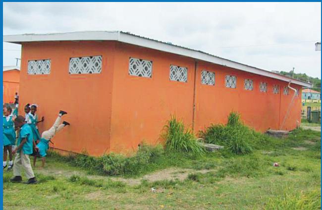
■ TOILET BLOCK - FUNCTIONAL, BUT IN NEED OF REPAIRS
