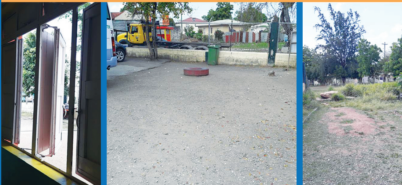
FIGURE 7.2: EXAMPLES OF AREAS FOR IMPROVEMENT (DAMAGED WINDOWS THAT PROVIDE INADEQUATE VENTILATION, MAIN ROAD AND UNPAVED SURFACES CONTRIBUTING TO DUST LEVELS, LACK OF FENCING IN SOME AREAS)
