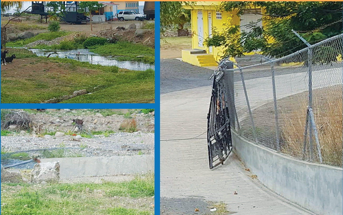
FIGURE 7.1: IMAGES HIGHLIGHTING AREAS WHERE PERIMETER FENCE AND GATE REQUIRE REPAIRS (MAY 2019)
