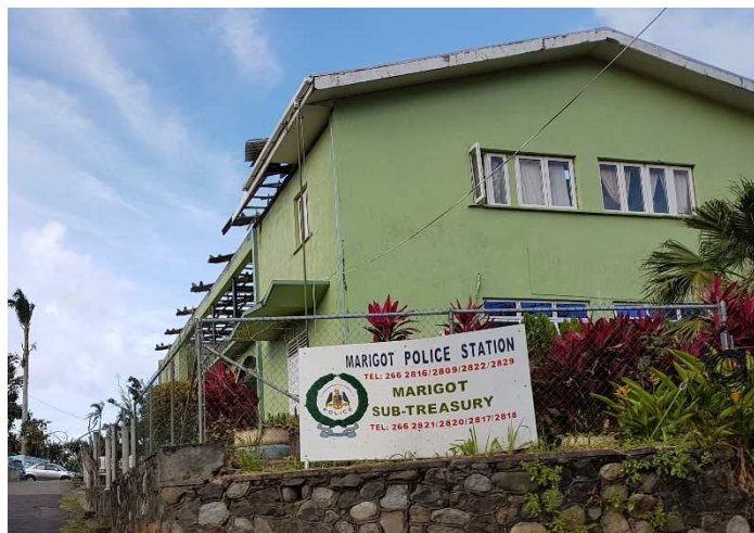
Marigot Police Station roof needing repairs. Dominica. March 2018.
