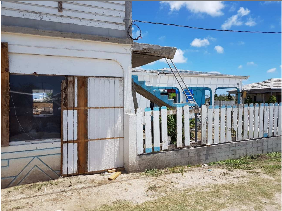
'Bus Stop Guest House' and 'Lynton's to Go' takeout snack bar, undergoing renovation. Barbuda, April, 2018.
