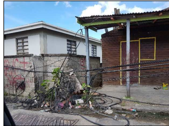
Downed power lines in Salisbury, six months after Hurricane Maria. March 2018.
