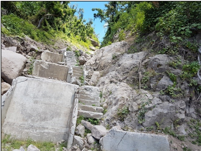
A damaged portion of the Waitukubuli National Trail. March 2018.
