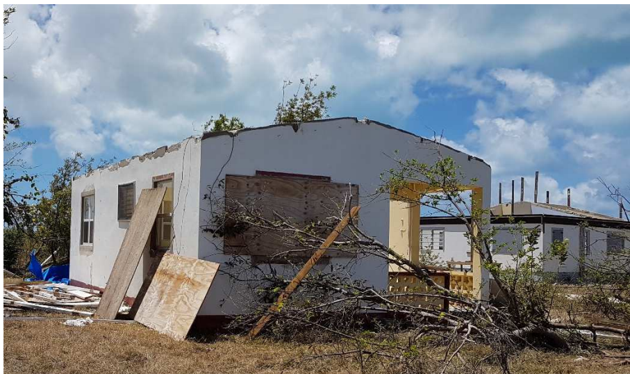
Remnants of a home in Codrington, Barbuda, April 2018
