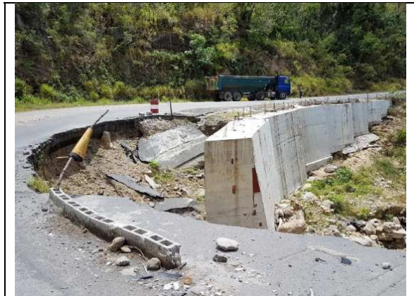
Major roads damaged by erosion caused by torrential rain from Maria. March 2018.
