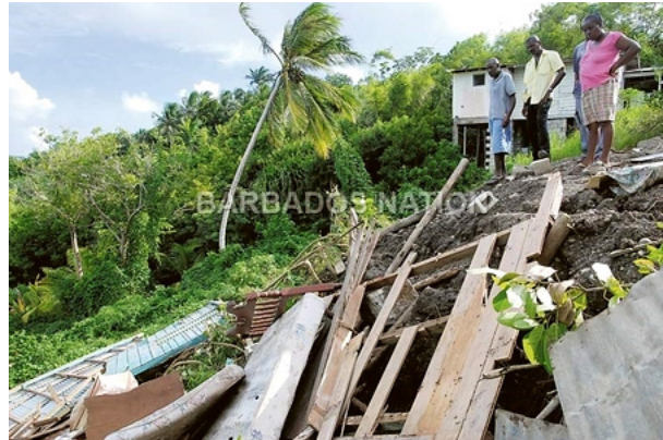
FIGURE 3: RESIDENTS LOOKING AT THE MANGLED HOUSE WHICH COLLAPSED AS A RESULT OF THE INSTABILITY OF THE LAND.
