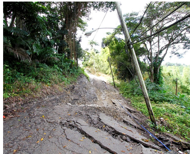
FIGURE 11: COLLAPSED ROAD IN WHITE HILL, LAND SLIPPAGE AND LEANING UTILITY POLES
