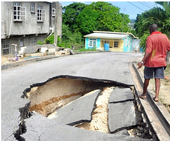
FIGURE 10: PART OF A COLLAPSED ROAD AT SOUTH DISTRICT IN ST. GEORGE
