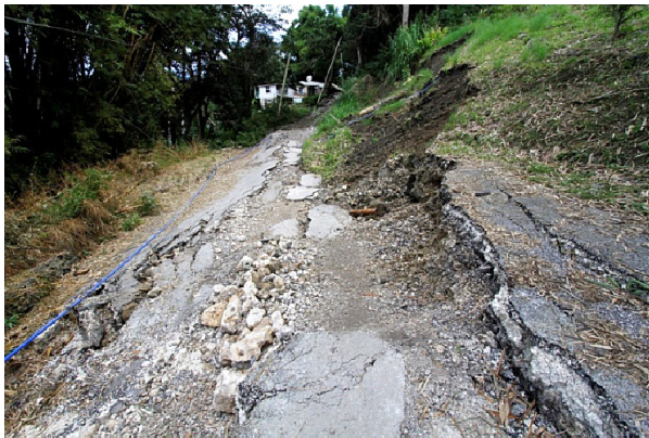
FIGURE 2: LAND SLIPPAGE IN THE SCOTLAND DISTRICT
