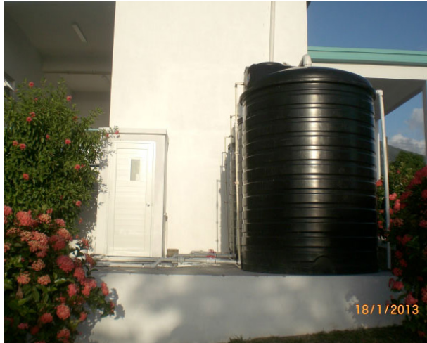
FIGURE 12: NEWLY INSTALLED 1,000 GALLON WATER STORAGE TANK
