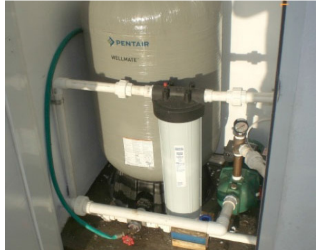
FIGURE 13: NEW PUMP ROOM WITH PUMP AND WATER FILTER SYSTEM
